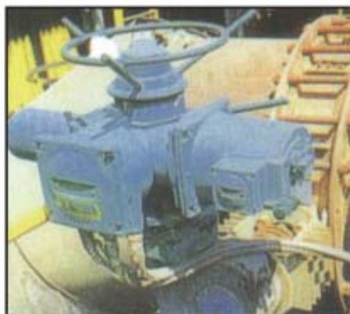
1400 mm valve in operation in a platinum smelter
